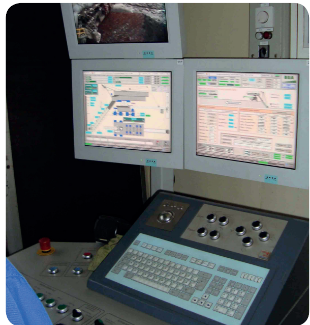
Image 3: All relevant data from the diagnosis and the visualization systems are centrally displayed at the control room.
