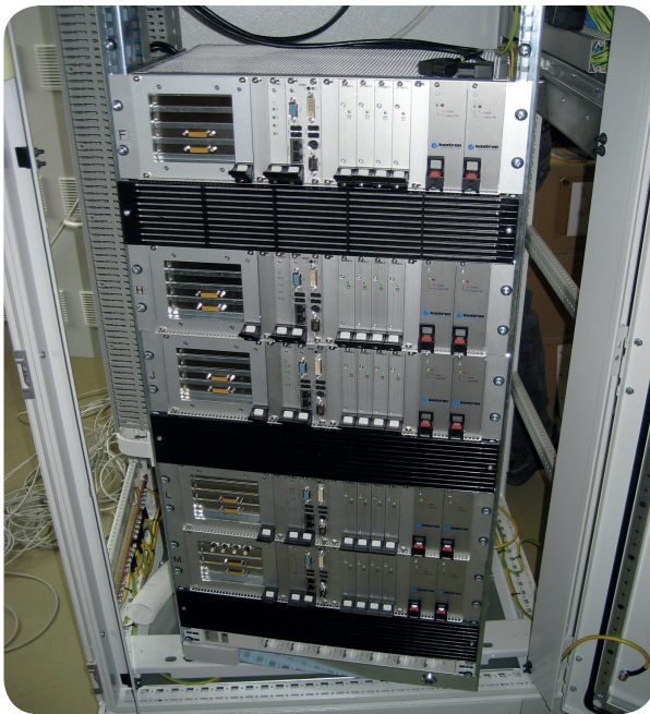
Figure 1: The VDEC units in the control room.
