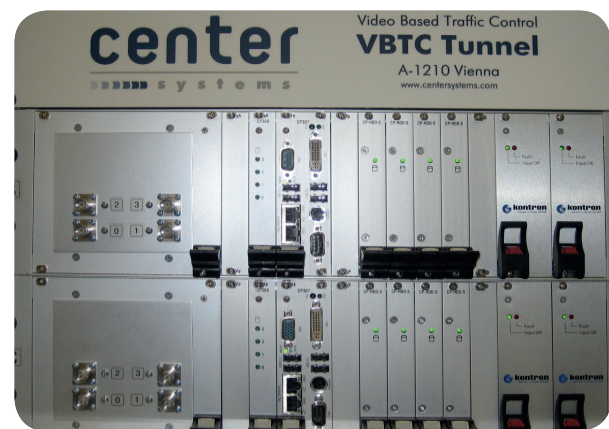
Figure 4: How VBTC Tunnel's VESA units are constructed, from left to right: PCI-based frame grabber cards, a RAID controller, a Kontron CP307 CPU board, four hard-drive slots, and two power supply units
